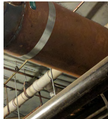
Basement mechanical space
